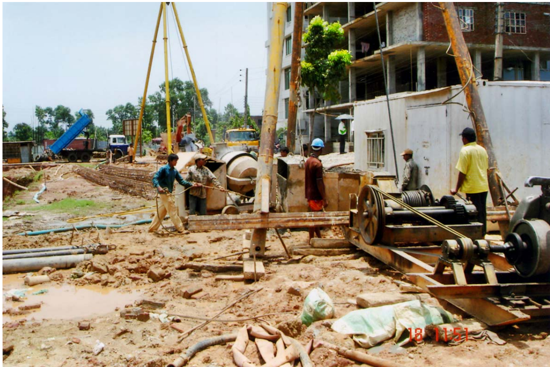
Machines seen on the picture will be sued for concocting construction materials for the 14-storey DSE building.
