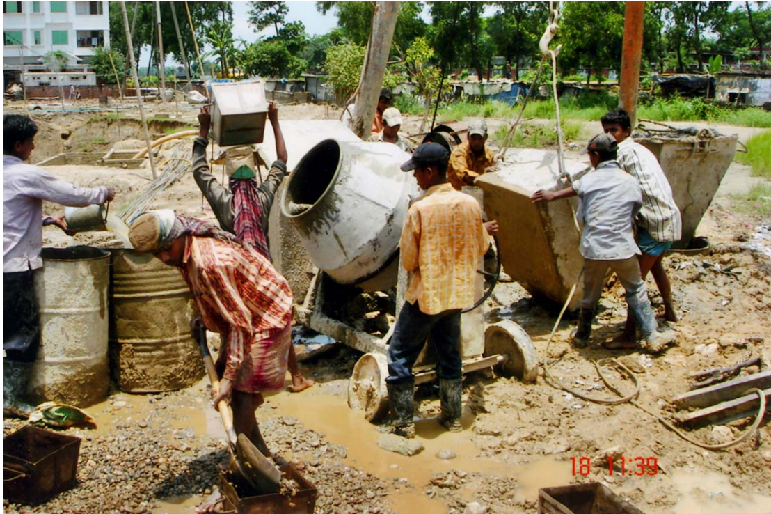
Workers-breaking brickbat, pouring water into drum containing construction materials and carrying materials on the ground of the DSE building (under construction).
