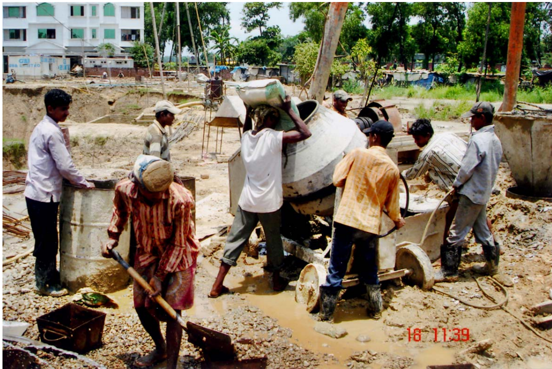
A man engaged in DSE building construction work is pouring brickbats into rolling machine for the final use at DSE building.
