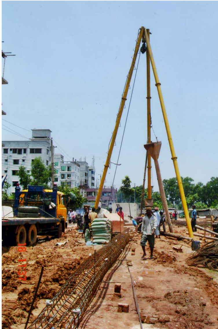
Workers, rod, cement and truck are seen on the picture-all will be used for the construction of DSE building.
