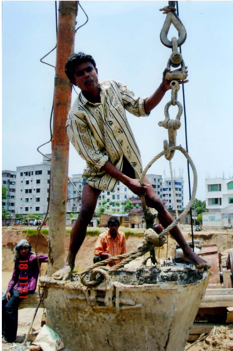
A worker is toiling to concoct construction materials, which will be used at DSE building construction work.
