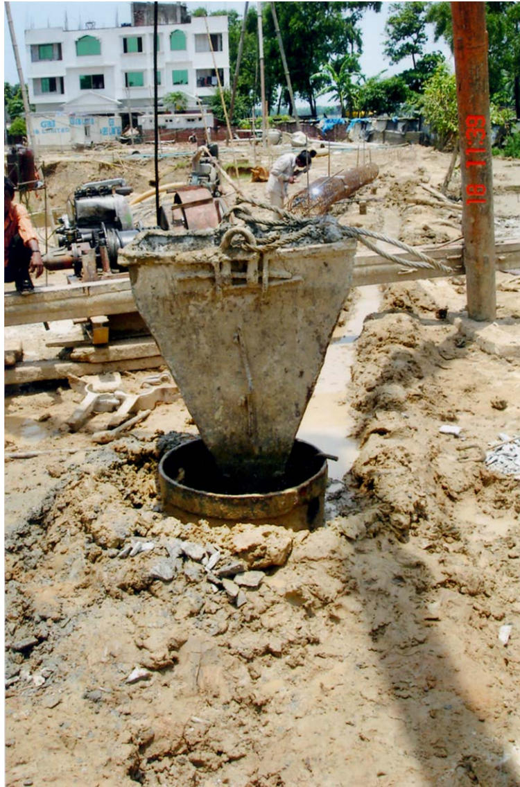
A worker is seen working beside whom a big tub containing brickbat, sand and other construction materials has also been kept.
