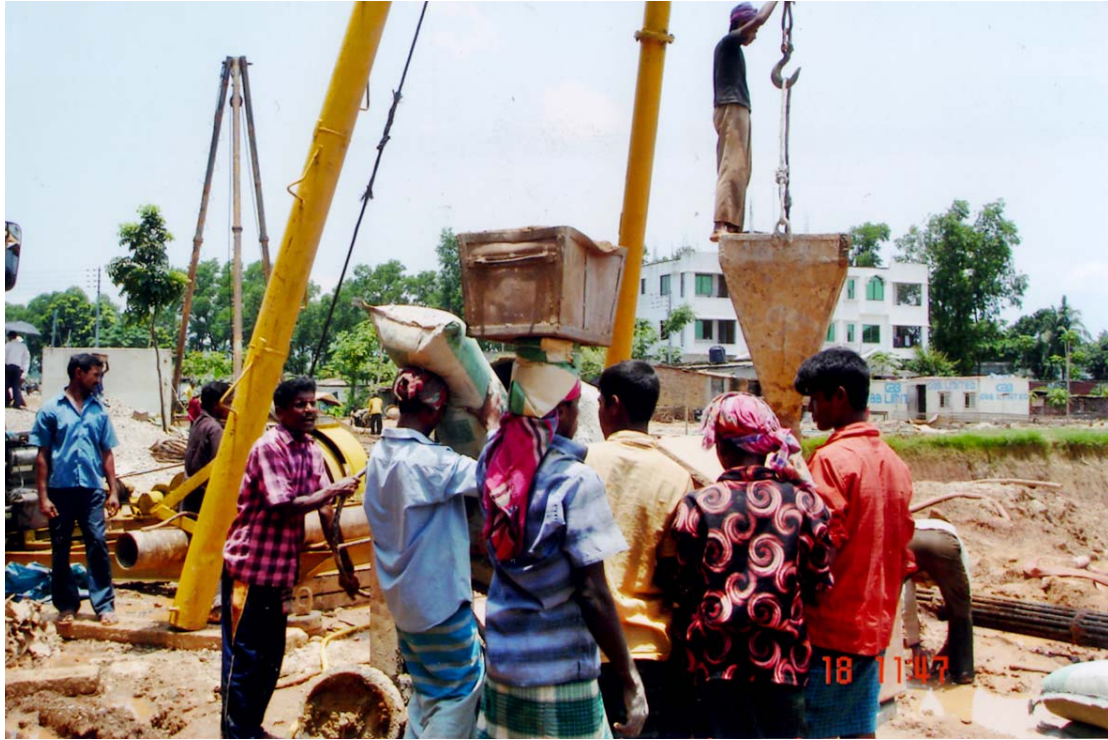
Workers-someone is carrying cement on head, someone digging hole and others are in another jobs at the DSE building construction work at Nikunja, Dhaka.
