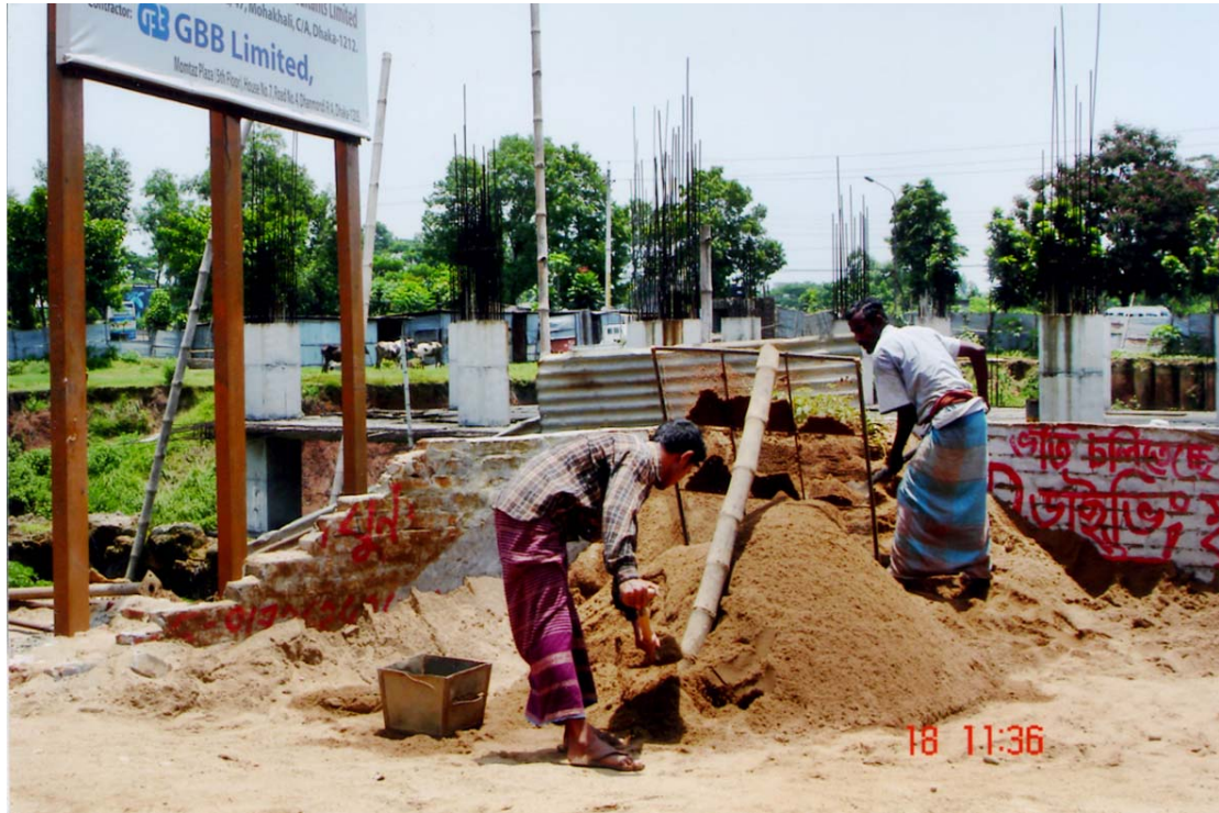
A worker is filtering sand, which will be used for the construction purpose of the 14-storey DSE building.
